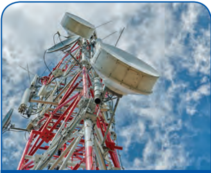
Telecom -Data Infrastructure
