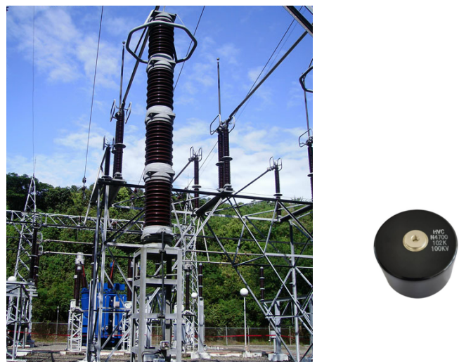
Power Electronic Equipment
