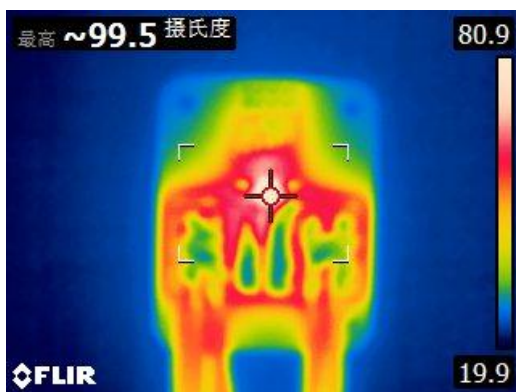
Package Thermography (Input Current 40A)
